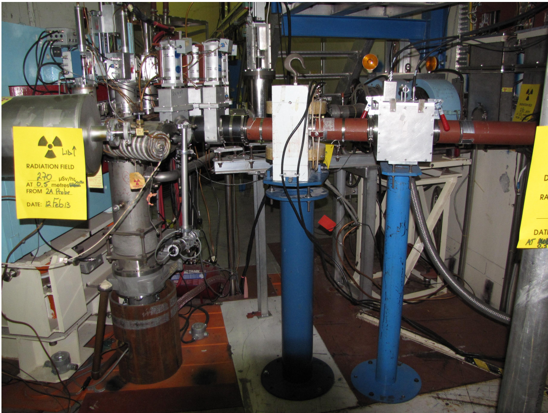
Figure 2: Photo showing the switching magnet, isolation valve, steering magnet and diagnostic box (from left to right) in the existing 2C4.
